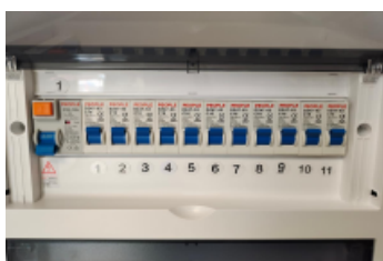
Main circuit breaker panel
