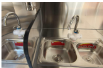
Double sinks + hand wash sink
