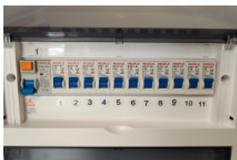
Main circuit breaker panel
