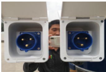
2 x outside power inlets (16A or 32A)
