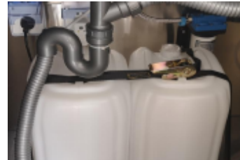
25L clean water tank & 25L waste water tank
