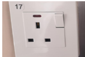
12 x inside UK power sockets (UK style)
