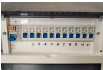
Main circuit breaker panel
