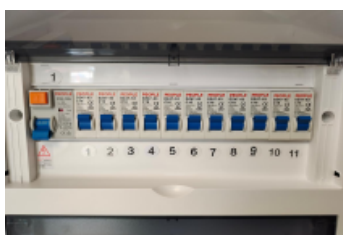
Main circuit breaker panel
